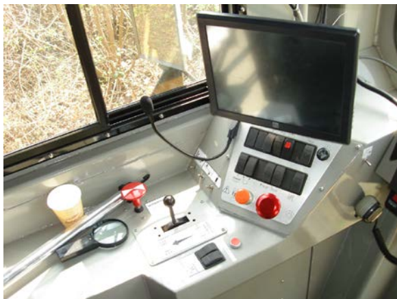
Main Operator's Console
