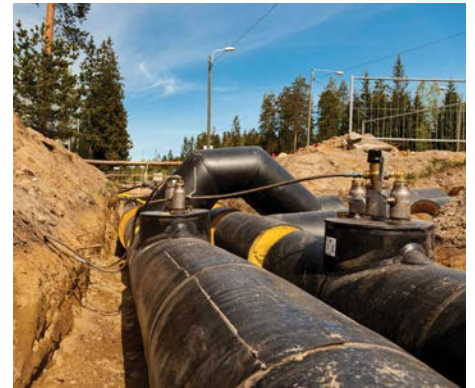
District heating pipeline.
