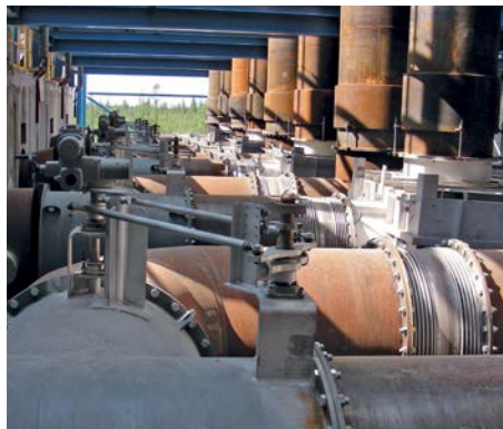
US-types installed in a flue gas system.
