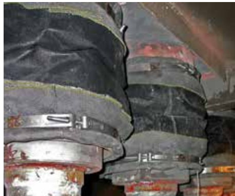
Flexgen expansion joints installed as pipe penetration seals.
