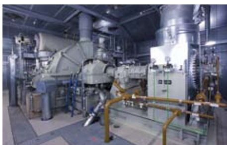
Steam turbine, lignite-fired power plant
